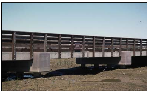
A new bridge was built to allow a path for bird watching and recreation.
