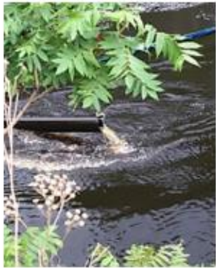
Photo 14: Jay Cooke State Park—water main break.
