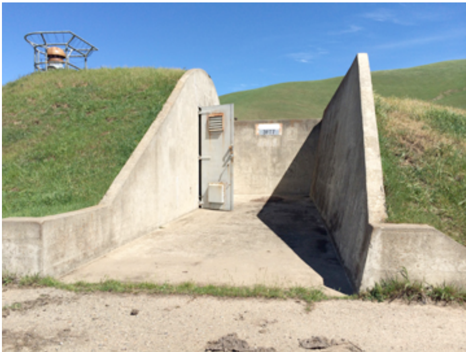
Typical Magazine: view of blast deflection and entry area, as well as earthen roof covering
