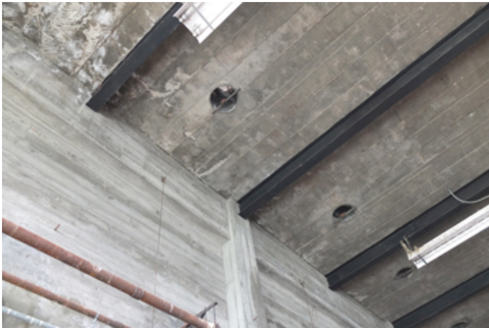
Building 1A-24: detail of ceiling showing efflorescence
