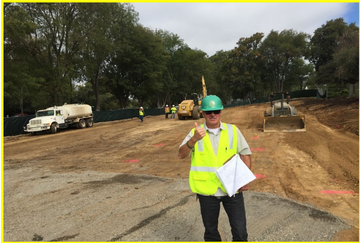
View of the parking lot in progress inspected daily by our project manager Colin Ross.
