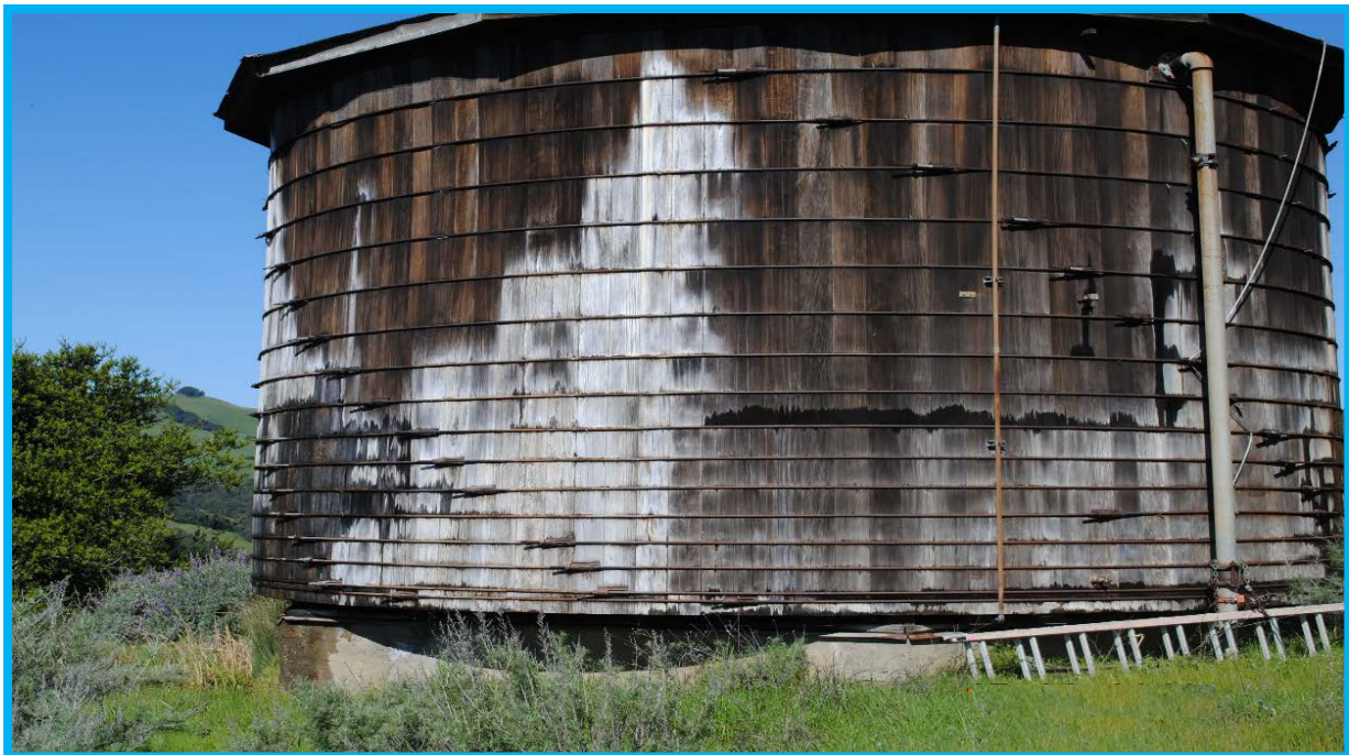
Current water tank that needs replacing.
